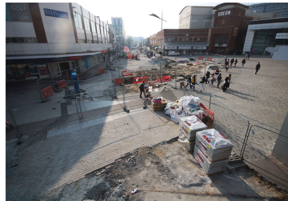
Figure 24: Major construction works in Southend-on-Sea as part of the SUNRISE co-implementation phase. The thorough co-creation process also helped to mobilise additional regional funds. © City of Southend-on-Sea.
